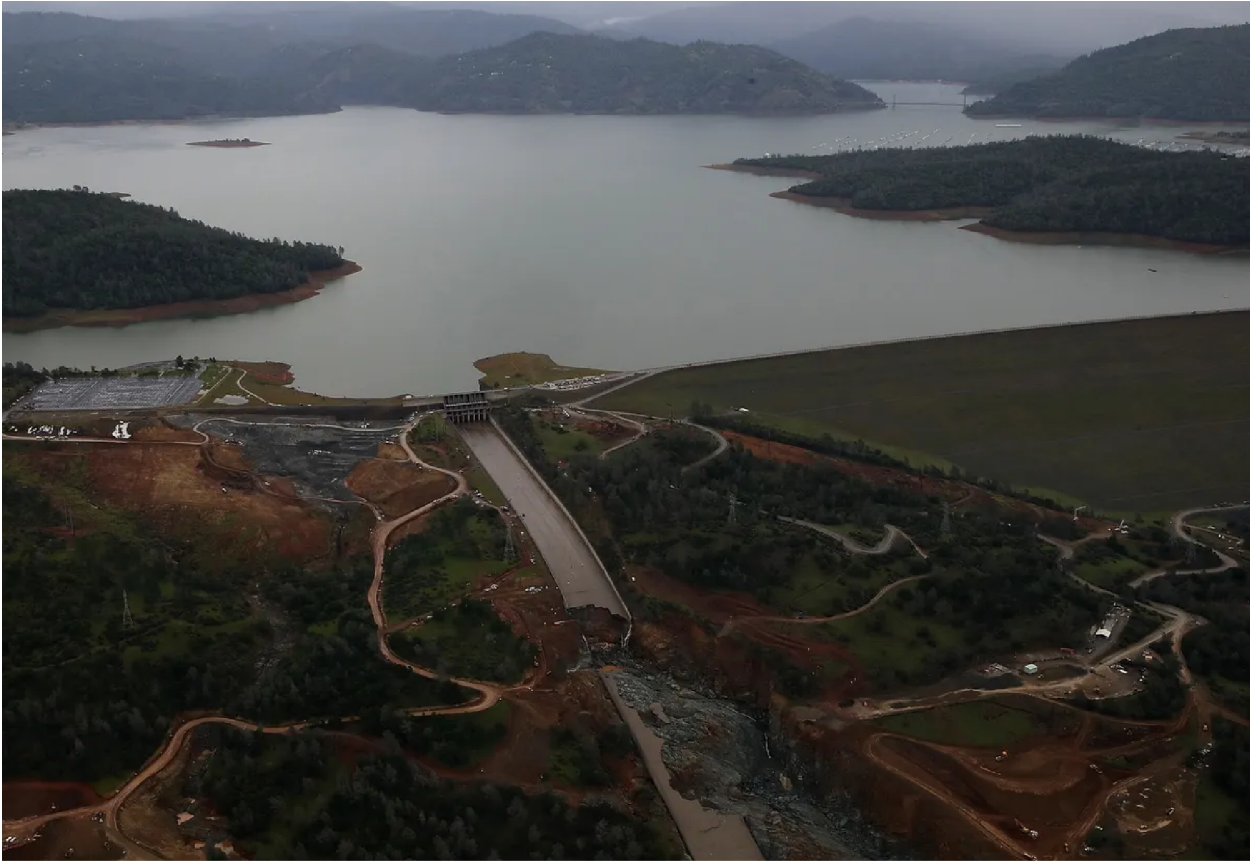
The heavily damaged spillway at Lake Oroville in Oroville, California, in 2017. Photographer: Justin Sullivan/Getty Images
