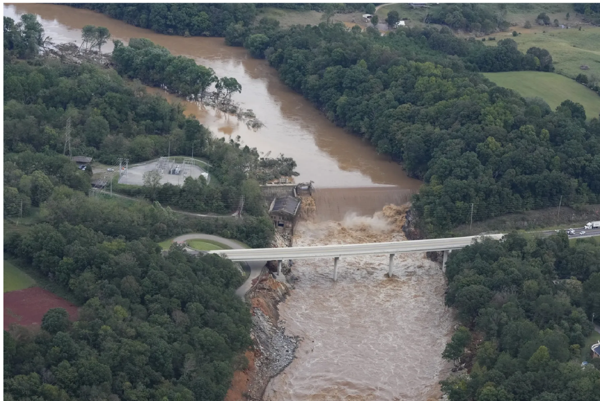
The Nolichucky Dam in Greene County, Tennessee, following Hurricane Helene on Sept. 28. Photographer: George Walker IV/AP Photo
